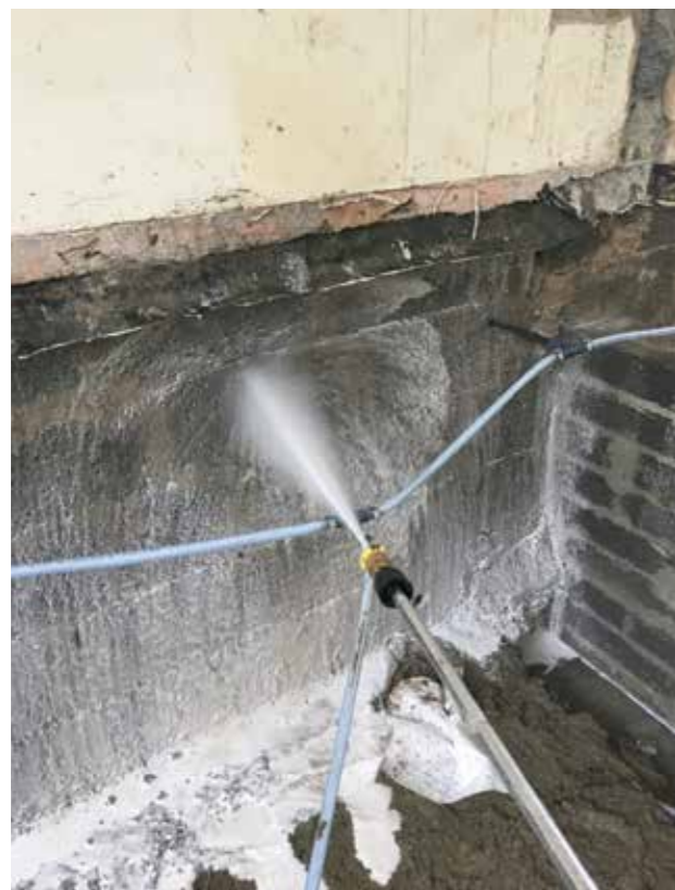
▲ Figure 6. Treatment to the exposed blockwork inside the property. (© Avada Environmental Ltd)
