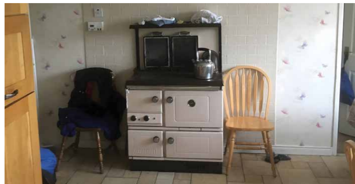
▲ Figure 3. AGA cooker, the source of the kerosene leak. (© Avada Environmental Ltd)
