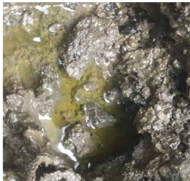
▲ Figure 7. Free product at property foundations. (© Avada Environmental Ltd)
