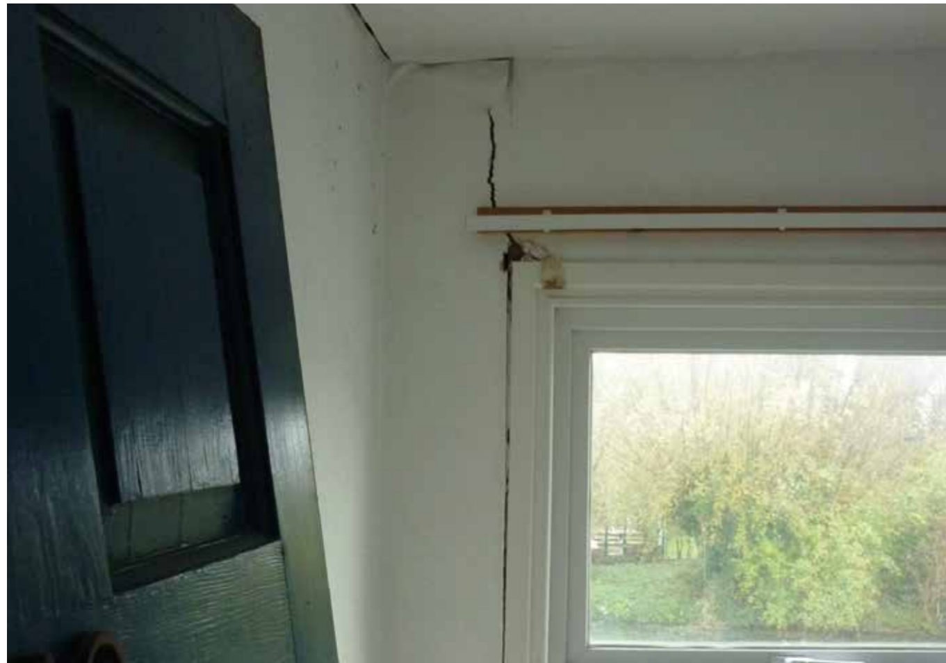
▲ Figure 1: An example of minor building damage caused by subsidence. (© RSK)
