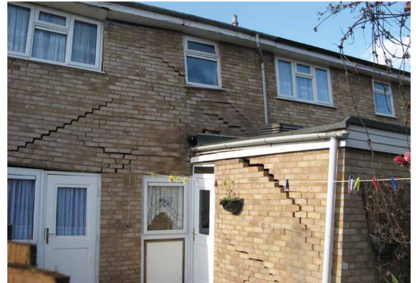
▲ Figure 2. Damage to housing caused by a sink hole. (© RSK)
