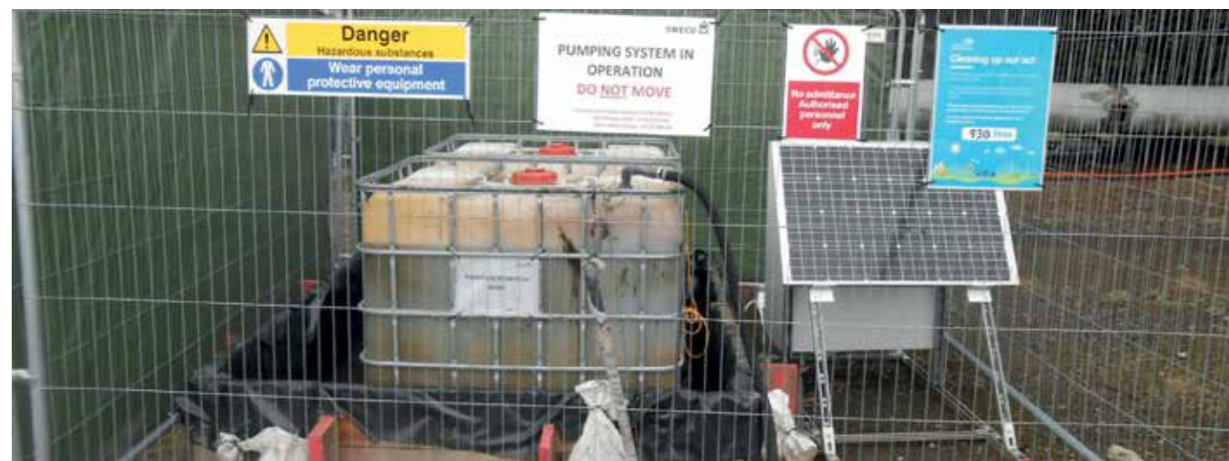
▲ Figure 4. Remediation pumping system for well BHS17-04A (© Tim Vickers).
