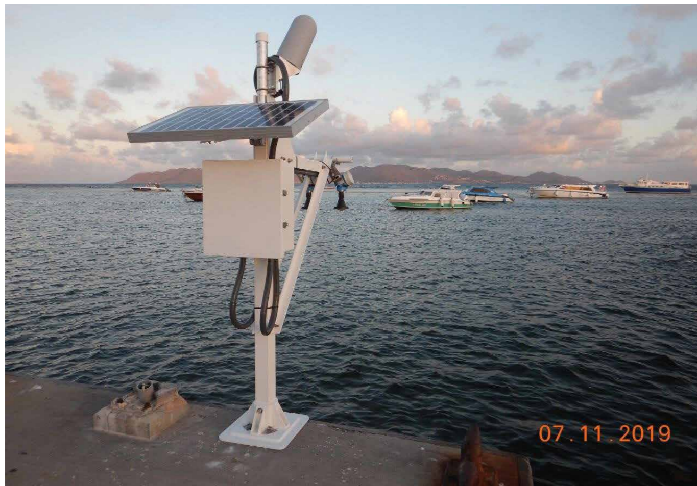
▲ Figure 4. Post-hurricane remains of the Blowing Point tide gauge shown alongside the newly installed 'hardened' replacement system. (© Jerard Jardin, Jardin Sea Level Systems)
