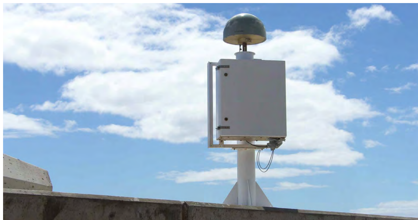
▲ Figure 5. A GNSS receiver installed at Ruperts Bay, St Helena. (© Alan Hudson)
