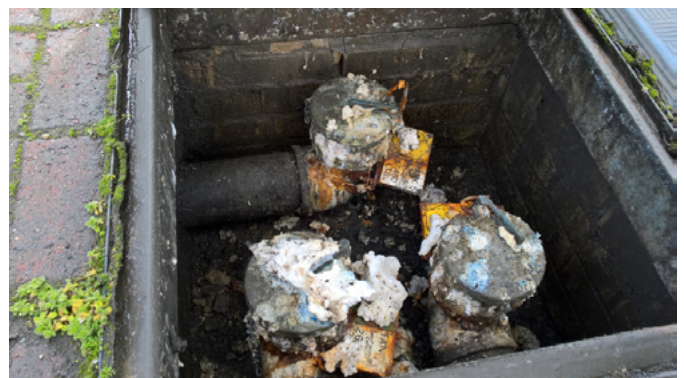
Figure 12: Disused fuel filling points with evidence of foam from tank infill
