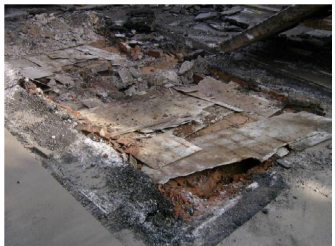
Figure 14: Asbestos sheeting found on site
